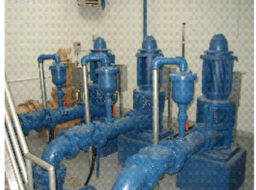
High Service and Backwash Pumps
